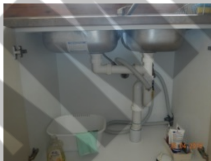
Damaged cabinets; sink leak
