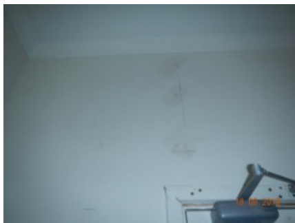
Wall affected by dampness - downpipe leak
